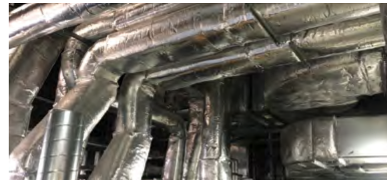
FI22 Ductwrap installed in a plant room at Royal Hobart Hospital.
